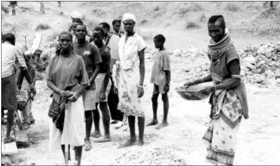
Teams of Samburu and Turkana women and men working together on constructing a sand dam
