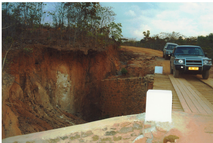
Figure 7. Erosion caused by the construction of a low-cost feeder road in the hills of northern Malawi (photo: K. Esser).
