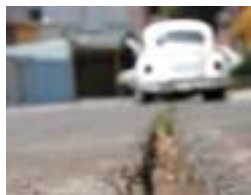
Inhabitant of the Izcalli District in the center of Ecatepec municipality – State of Mexico (Valley of Cuautitlan-Texcoco) complain about the deterioration of the highways caused by the natural gas network which has been constructed by the Mexigas Company. © Newspaper El Universal (Mexico) - Photographic Archives / Photographer: Luis Garcia Soto
